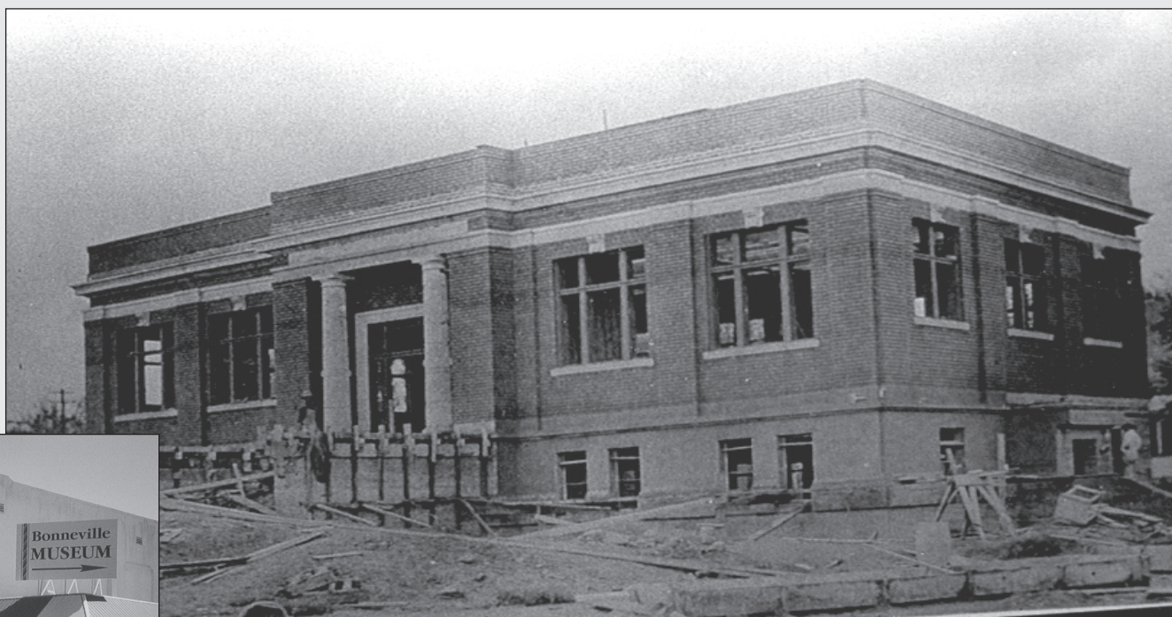
The Idaho Falls Carnegie Library under construction in 1916. The historically registered library served an ever-growing population until 1977 when a new, larger library was opened.
